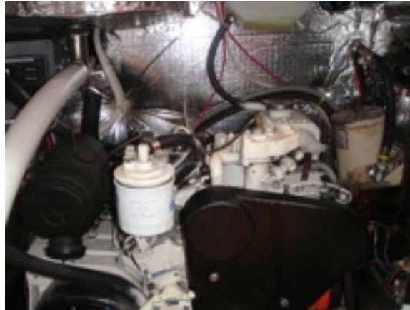
Existing Genset - 5.5 Kw NextGen Generator with 240v AC Output
