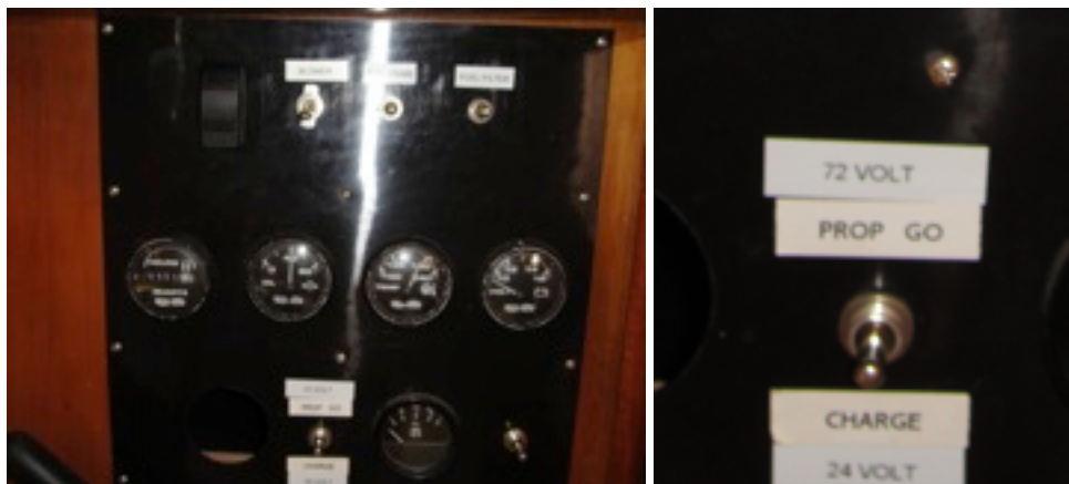
Genset and Utility Subpanel - (right enlargement) Control Switch for Battery Contactors
